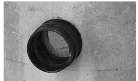
6. Installed EZ-Bell Adapter Coupling ready for service.
